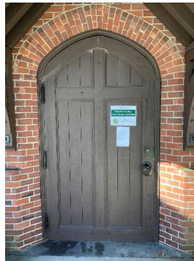
BE4 – The main door to Hadley Hall fits reasonably well, though there is a gap along the top arch.
