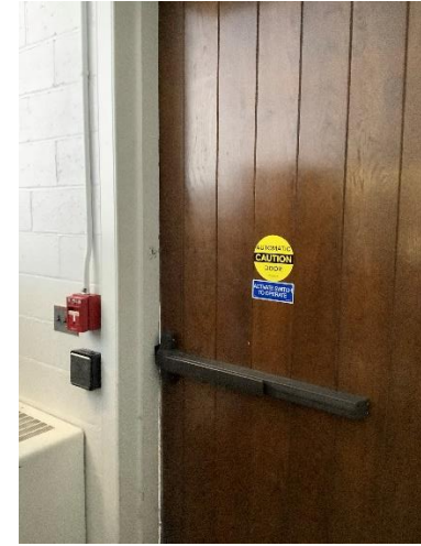
BE5 – This door in Hadley facing Church Street also shows a gap and air infiltration, especially below the panic bar.
