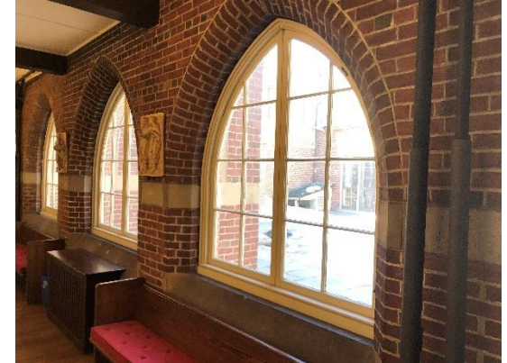
BE6 – Arched windows along the corridor are candidates for window inserts built as a parish work day.
