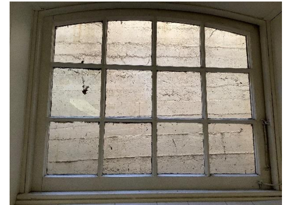
BE11 - This window is not operable and could be replaced with a double or triple pane fixed unit.
