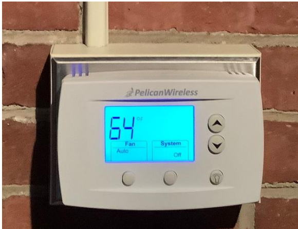
B1 – Wireless thermostat in Sanctuary provides a more modern control in the existing heating system
