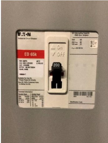
H8 For heat pumps, it is likely additional electric capacity will need to be added to this 200 amp panel and the 125 amp panel in H9.
