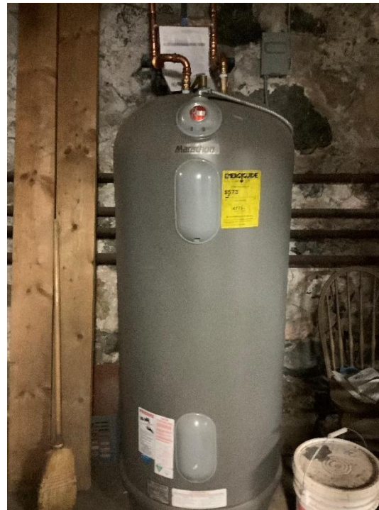
H10 – This 91 gallon hot water heater serves the entire building.
