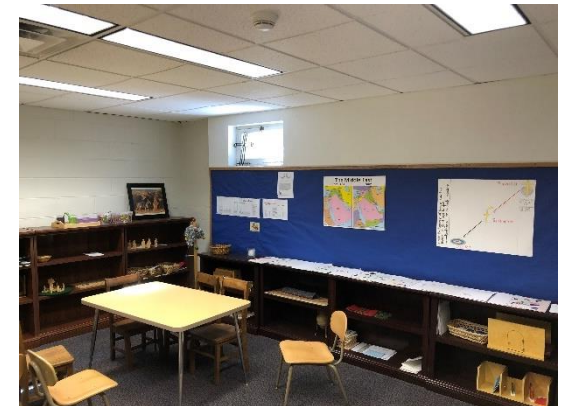
BE12 - The hopper style window is currently operable but could be replaced with a fixed unit.
