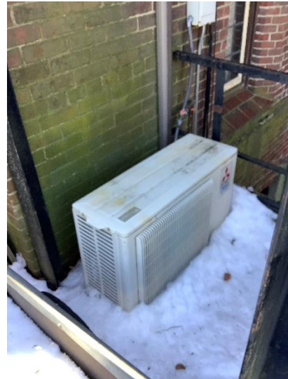
H6 - Heat pump for the Rector's office.
