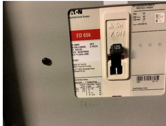
H9 – 125 amp electric panel
