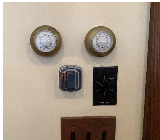
B5 – Chapel thermostats, apparently one controls the daytime temperature and the other nighttime – but how they are coordinated is unclear.
