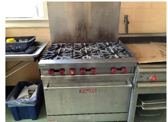
E6- Kitchen range – gas pilot flames always on
