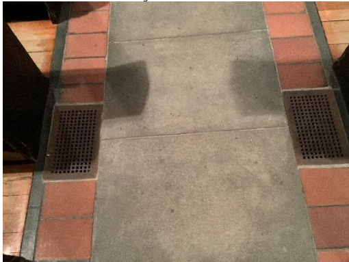
H4 - Hot air grates in the Sanctuary floor bring warm air up from undercroft tunnels.
