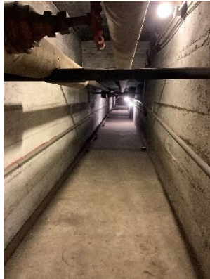
H3 - The undercroft tunnels provide another path for heat to be distributed to the Sanctuary via the grates in the floor in Photo H4. The high temperature in these tunnels indicates how inefficient this system is.
