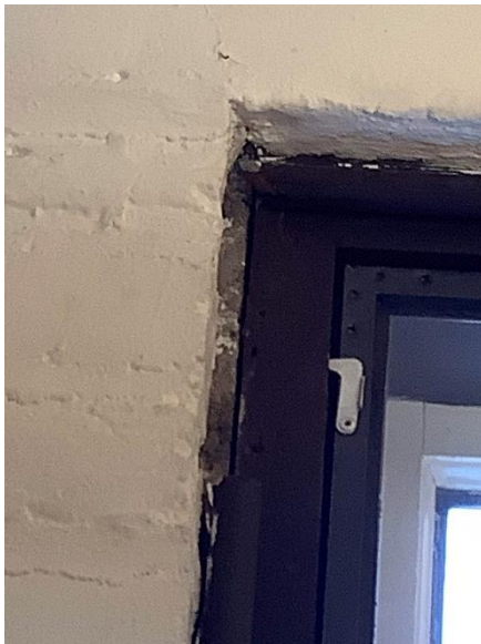
BE2 – There is no caulk between the window frames and the walls, allowing air infiltration.
