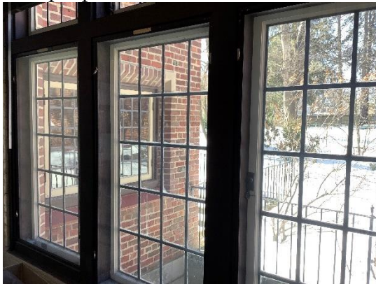
BE8 - The window at left has a window insert while the others don't, although the clips on the frame suggest inserts did exist at one time.
