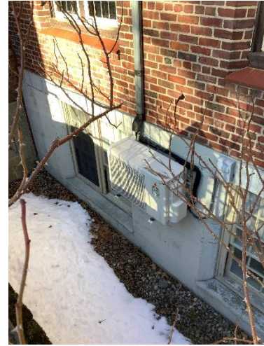
H5 - Heat pump for the main office.
