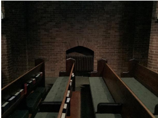
H2 – Radiators like this one in the Sanctuary are common in the building.
