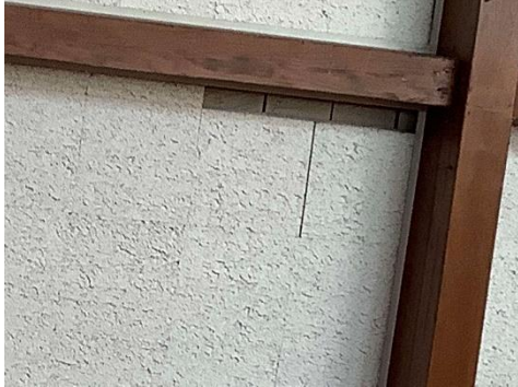
BE1 – This gap in the acoustic tile appears to show the roof sheathing, indicating no insulation.
