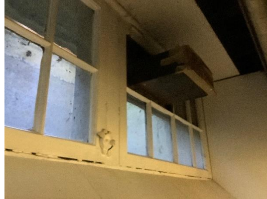
BE10 - This basement window appears to have been used as a vent but now is a candidate for replacement
